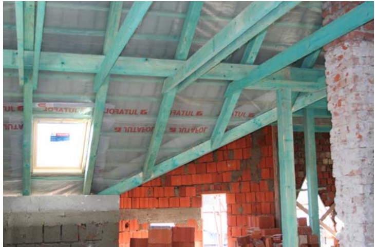
Insulation being put into the new roof over the sleeping quarters for the seminarians.
